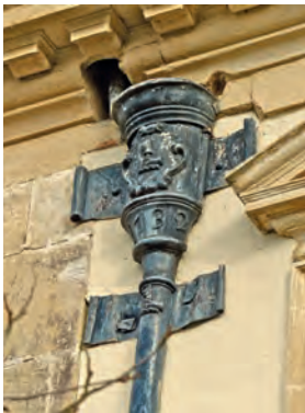
Fig. 5b Shepton Mallet, Bowlsh House, Rainhead dated 1732 and bearing the Howe crest
