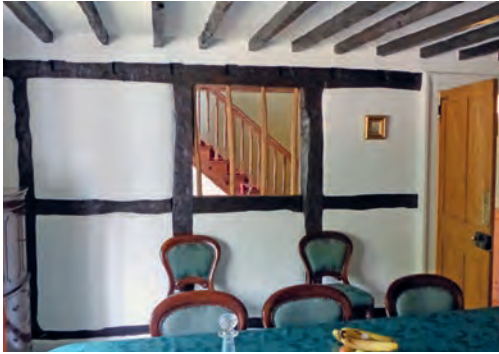
Fig. 1b Chedzoy, Westfield Farm, Wattle and daub panels to an oak-framed partition
