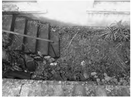
Fig. 8 Derelict basement in Bath
