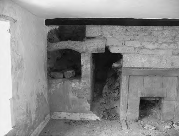
Fig. 7 Old Harp House, Over Stratton, remains of bressumer and access to curing chamber
