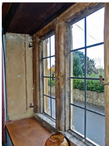
Fig 11 South Petherton, The Old Granary: 17 th -century ovolo-moulded stone window with shutter pintles and security bar brackets
