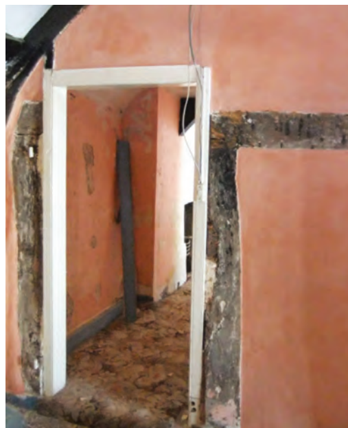
Fig. 1 11 West Street, Dunster: infill truss with evidence of earlier door to solar
