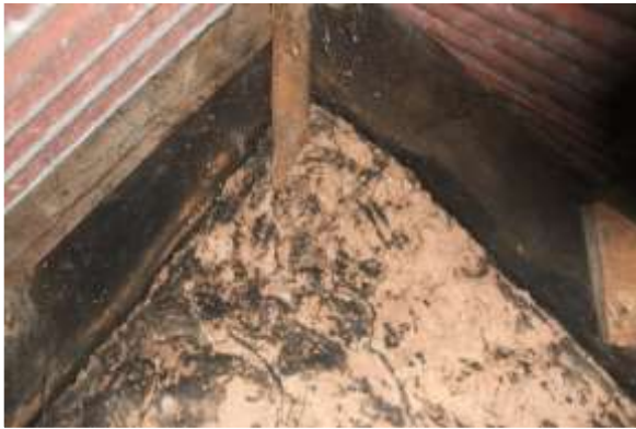
Smoke blackening to cruck roof with infill panel
