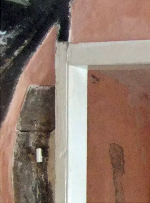
Fig. 7 Remains of solar door frame with pintel
