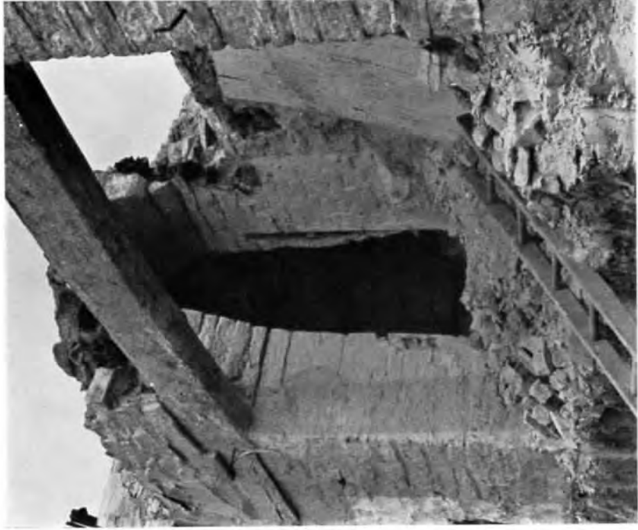
Plate 2. Type 2 chamber fully open to the hearth at a house in Wranitage.
