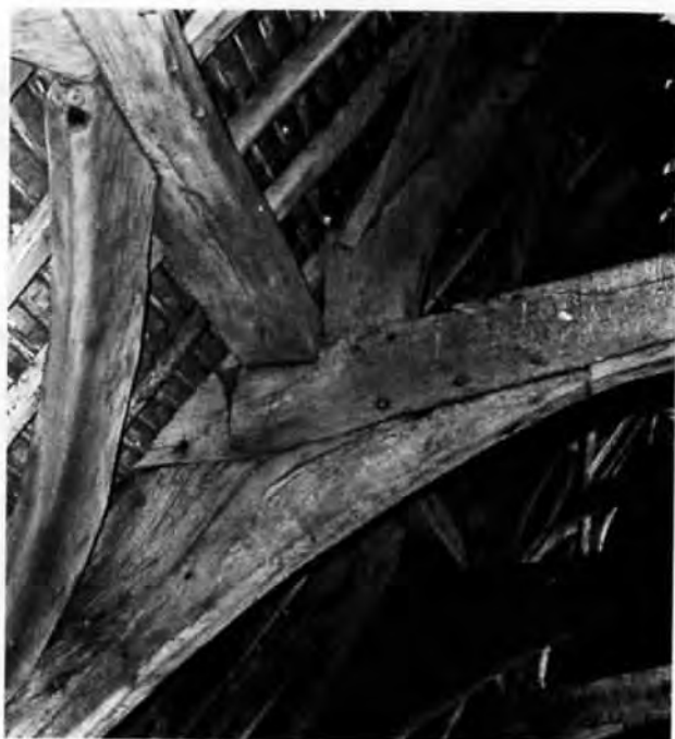
Glastonbury Abbey Barn Junction of base cruck, tie beam and roof plate
