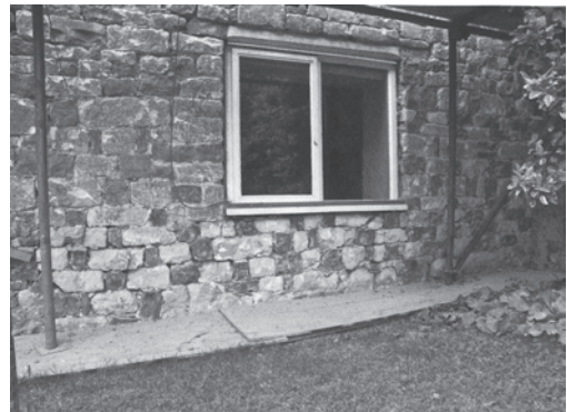
Fig. 2 Combe St Nicholas, Chequerwork on the front wall at Fforden (photo John Rickard)
