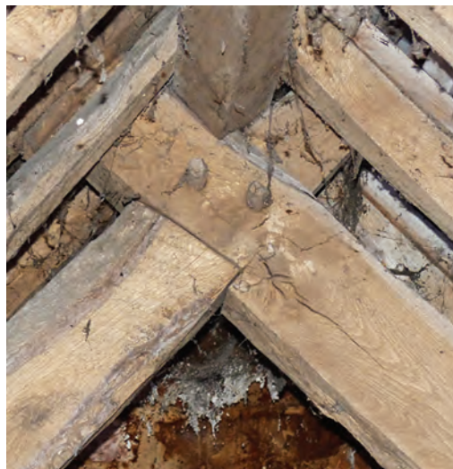
Fig. 13 Devon, Tytherleigh, Chard Rd, Penny Cottage & 2, Pinney Cottage, the halved and pegged truss apex
