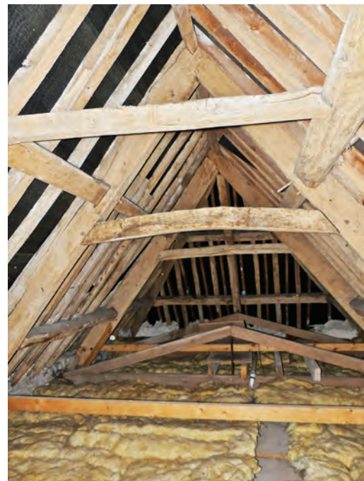
Fig. 3 Doulting, King's Rd, Hurlingpot Farmhouse, the roof trusses and the shallow hoist truss
