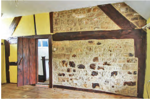
Fig. 2 Donyatt, Chard Rd, Thatchers Pond Frame FIII and truss with masonry replacing a possible fire hood of wattle and daub
