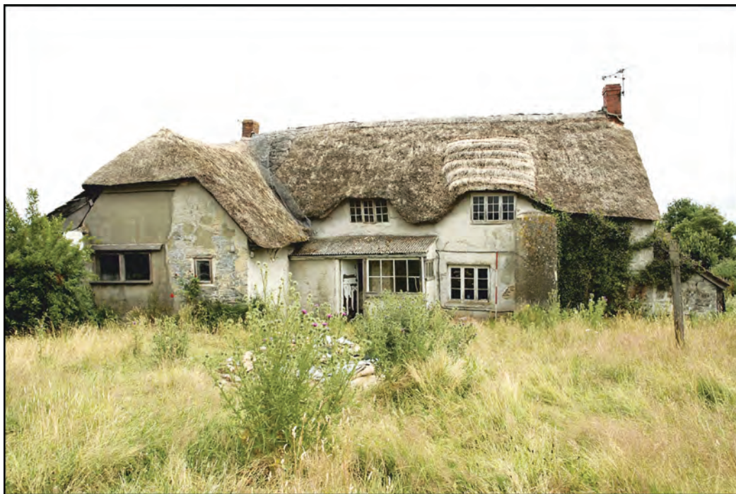
Fig. 2 View of the south-western (rear) elevation, with the rear-wing (left) and the modern buttress supporting the collapsing south-west wall (photo: Gary Young)
