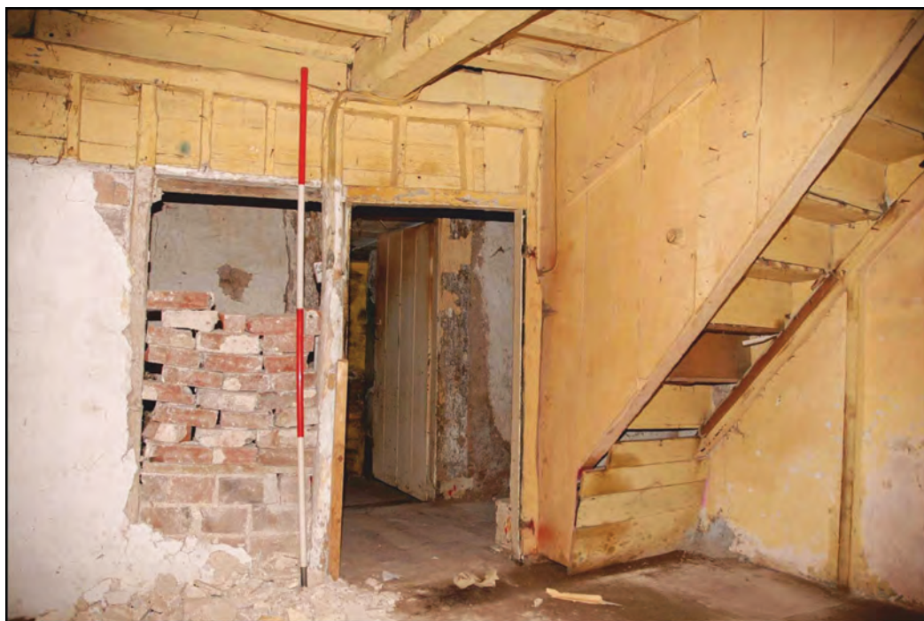
Fig. 9 The central room looking east, showing partition and well-made joists (photo: Gary Young)
