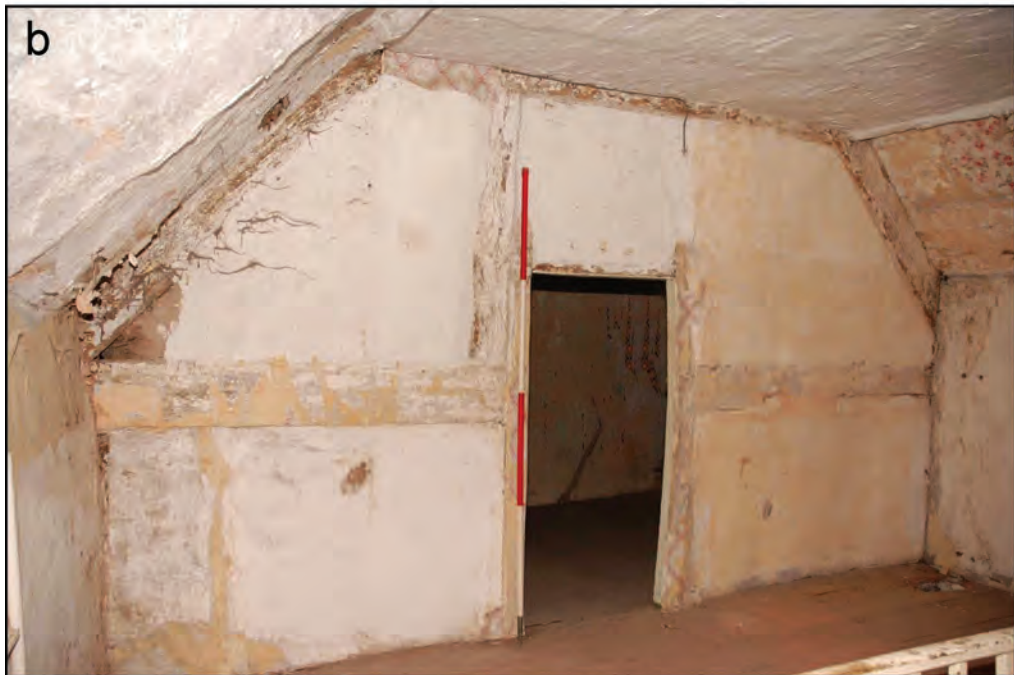
Fig. 11(a) Section 3, through the north-western end of the house, cut through the central room, showing the structure of the timber-framed partition defining the end room and the south-eastern elevation of the rear-wing (based on hand-measured survey by Exeter Archaeology). (b) View of the partition at first-floor level (photo: Gary Young)
