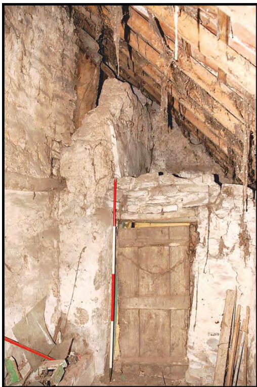
Fig. 4. View within the lean-to 'wood shed', looking west, showing the remains of the early cob front wall and the later timber partitions to the west (photo: Gary Young)
