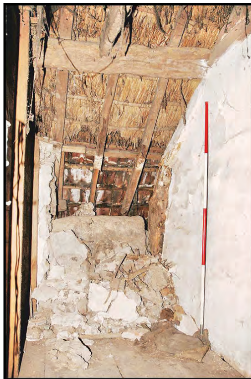
Fig. 5. View within the central first-floor room, showing the relationship of the roof and the original front wall, revealed by the demolition of the later timber partition to the outshut (photo: Gary Young)
