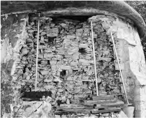
Fig. 2 The dovecote of The Grange, Woolavington. The collapsed west section in October 2005 (photo John McCann)
