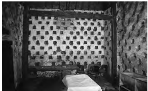
Fig. 8 Inside the dovecote of Church Farm, Trent, from the south (photo John McCann)
