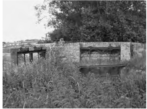
Fig. 3 Water control structures dated 1861 on the River Isle inlet to West Moor
