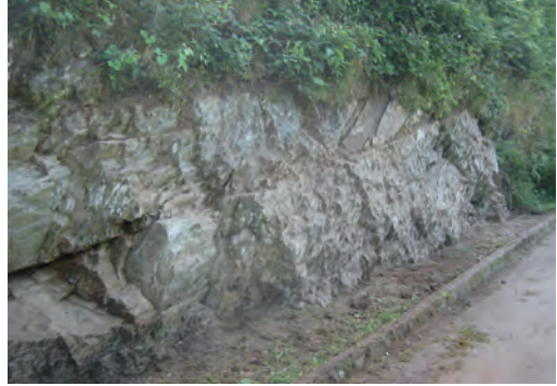
Fig. 4 The same LGS as in Figs 2 and 3, following completion of clearance work. Note a newly discovered fault-line, running from upper right of photo to lower left. There are now plans to install interpretation boards at the site to explain its geological interest (Photo: Garry Dawson)
