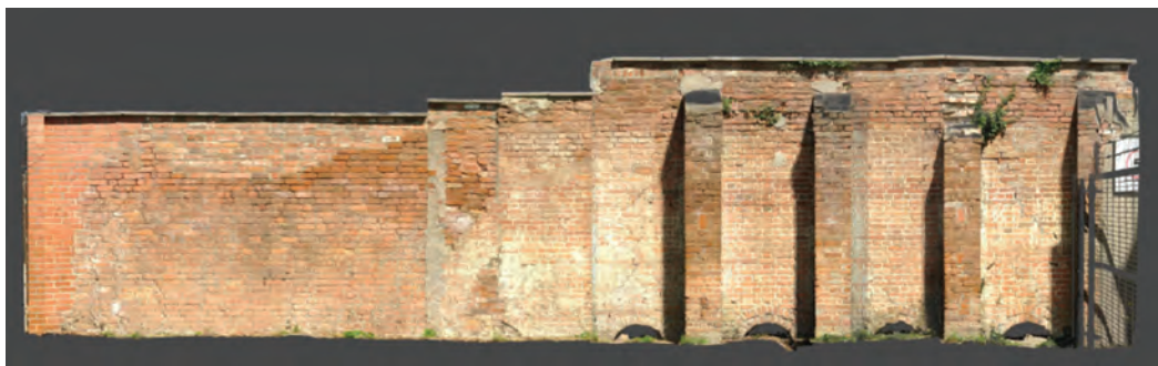
Fig. 4 Bridgwater, Bowrings Mill. Rectified image of kiln wall with fire mouths at base.
