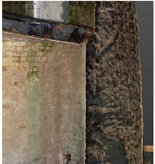
Fig. 6 Tile repairs to cracks in the ware chamber wall during conservation work in 2009
