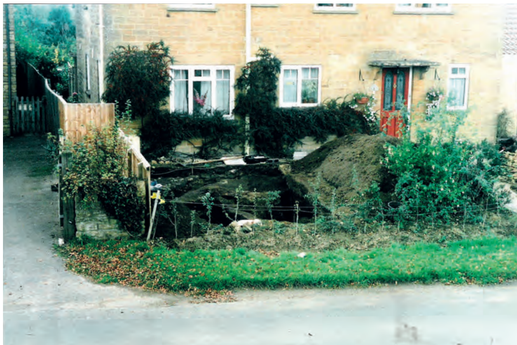
Fig. 7 Excavations in the garden of Sterton House, South Petherton. Looking west from Lightgate Road. The limited space for excavation is evident.
