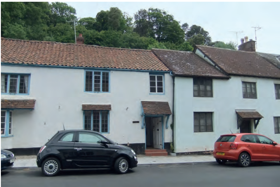
Fig. 8 Line of roof extending south under a different roof finish (at right of photograph)
