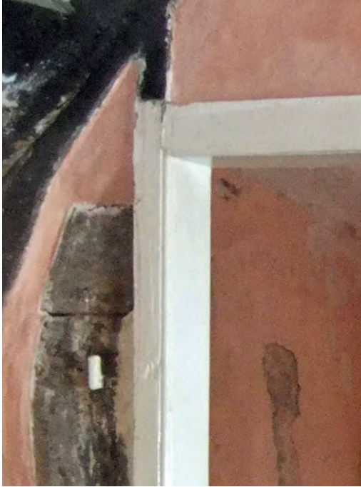
Fig. 7 Remains of solar door frame with pintel
