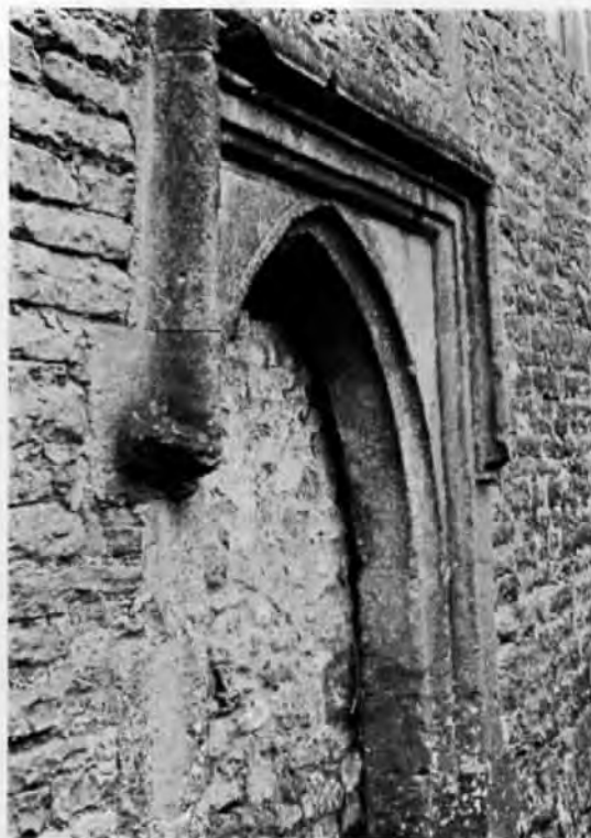
Plate 9. Manor House, Crocombe. Cross entry doorway of c.1400, hollow moulded two-centred head under angled dripmould.
