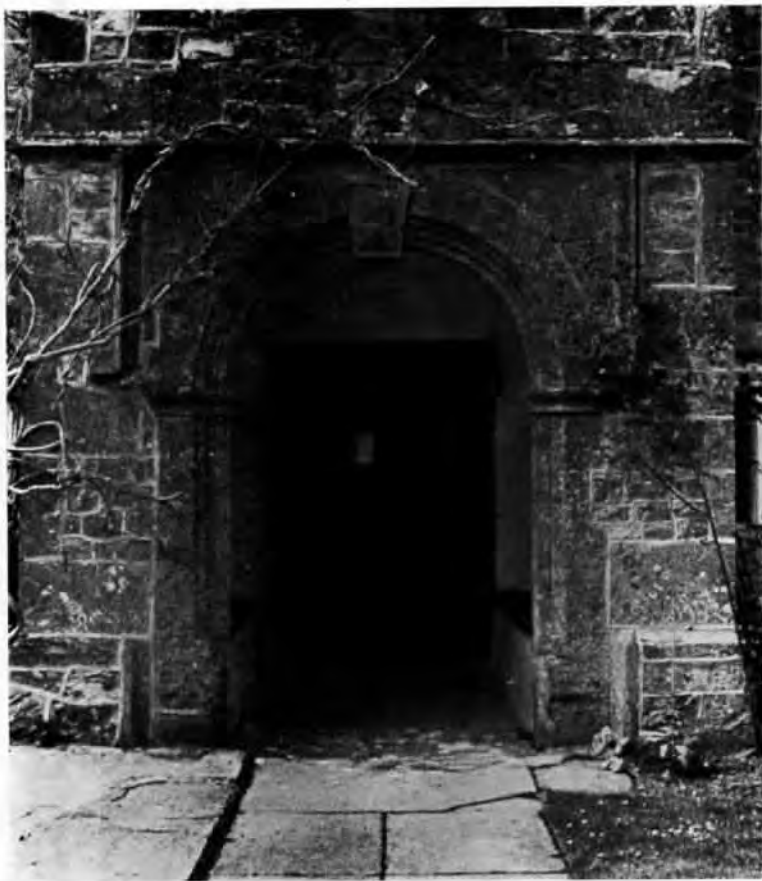
Plate 7. Weston Farmhouse, Combe St. Nicholas. 17C porch entrance with semi-circular head and dropped keystone.
