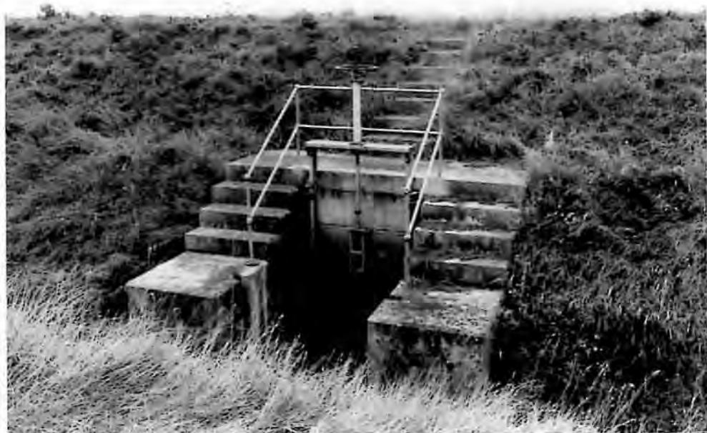
Plate 9 Small outfall (1990) at the western end of Wick Warth, viewed from the northeast.
